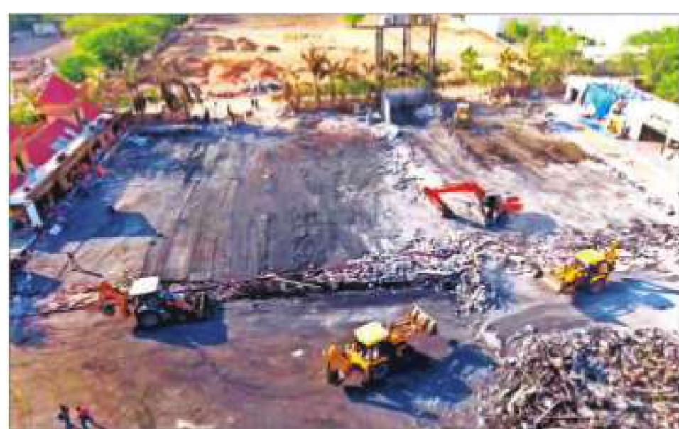
Debris being removed from the game zone site where a fire broke out on Saturday, in Rajkot, on May 27. At least 27 people were killed in the fire, according to officials.
